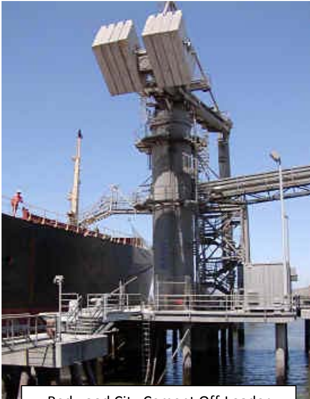
Redwood City Cement Off-Loader
